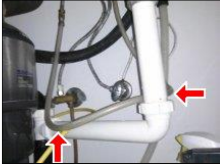
6.1 Item 1(Picture) kitchen sprayer hose leaking
