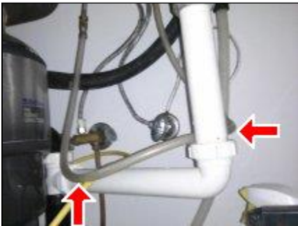
6.1 Item 1(Picture) kitchen sprayer hose leaking
