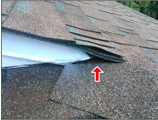
Possible leak. Needs to be calked.
